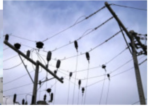
Fig 4 – b – Insulators and connections.
